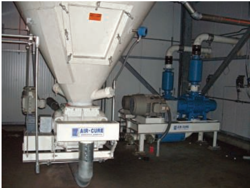
5. Dustless option. A dust hopper with a pneumatic conveying system. Courtesy: Air-Cure Inc.
