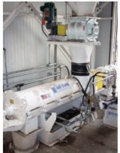
6. Wet and stick. A dust hopper with an agglomeration mixer. Courtesy: Air-Cure Inc.
