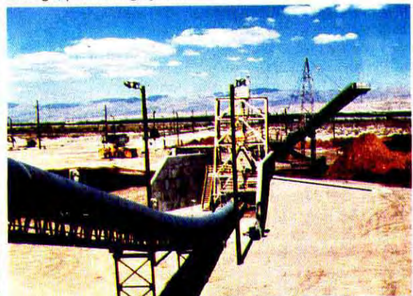
2. Processed fuel is supplied to boilers via receiving, storage, processing system
