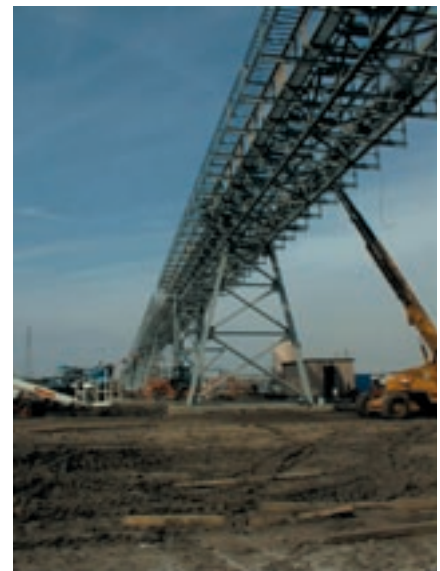
Fig. 7: Elevated section of the 4000 t/h, 3000 ft (915 m) long barge loading conveyor being constructed
